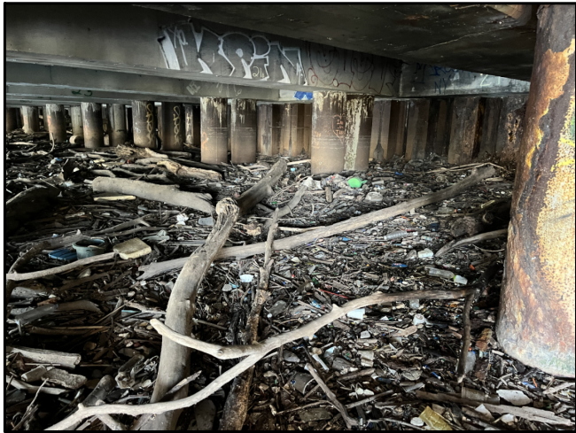
DEBRIS UNDER RELIEVING PLATFORM
