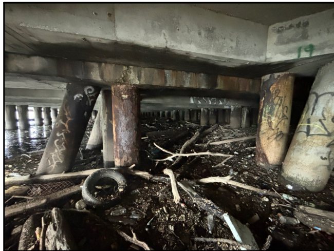
DEBRIS UNDER RELIEVING PLATFORM
