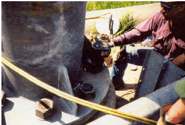
Figure 3. A Hydraulic Torque Wrench Tightening Anchor Rod Nuts to Achieve Needed Rotation.
