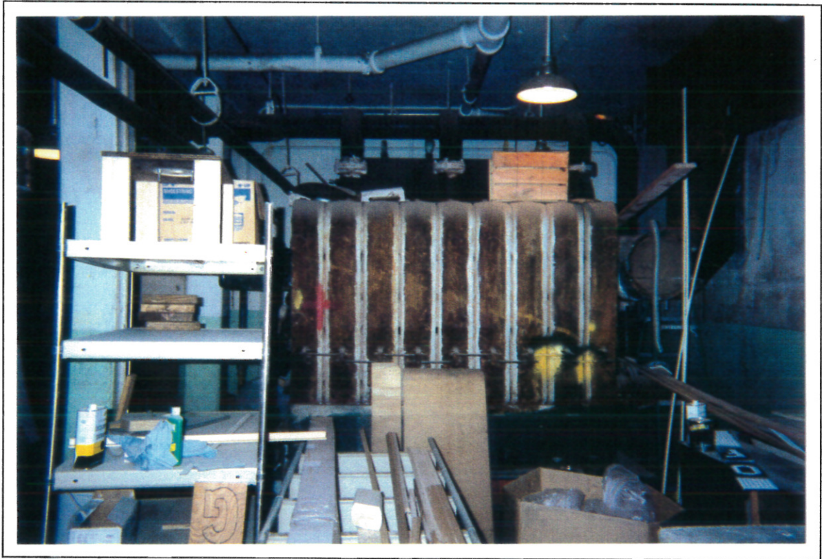
Photo 3: (Seneca Service Area (NYSTA) -Ontario County, New York) View of the side of the boiler in the basement. Notice the nine sections of the boiler. There is asbestos-containing material between the sections.
