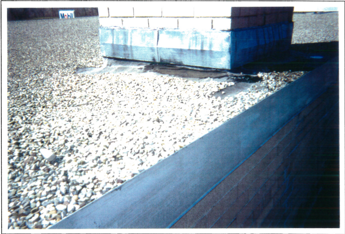
Photo 5: (Seneca Service Area (NYSTA) -Ontario County, New York) View of the asbestos-containing flashing around the chimney and the asbestos-containing built-up roof. This flashing is typical around the perimeter of the roofs and the roof top mounted units.
