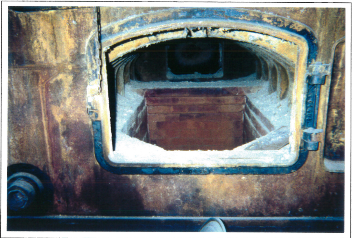
Photo 4: (Seneca Service Area (NYSTA) -Ontario County, New York) View of inside of the boiler in the basement. There is asbestos-containing material behind the black flanges of the doors. Additionally, the powdered material inside the boiler should be considered to be asbestos contaminated.
