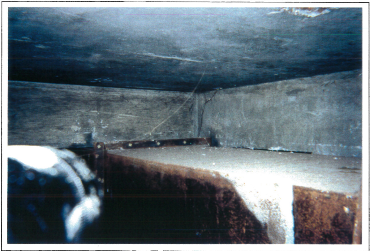
Photo 2: (Seneca Service Area (NYSTA) - Ontario County, New York) View of the asbestos debris on top of the chimney duct in the basement.
