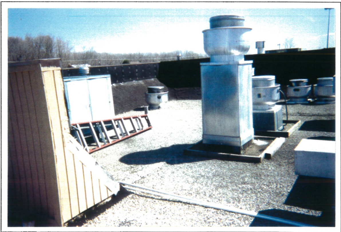
Photo 6: (Seneca Service Area (NYSTA) -Ontario County, New York) View of the asbestos-containing sealants over the nails in the rolled roofing (background along top of parapet wall) and the asbestos-containing built-up roof.
