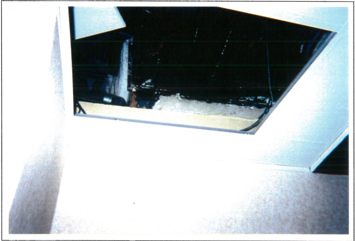
Photo 1: (Seneca Service Area (NYSTA) - Ontario County, New York) View of the asbestos-containing insulation on sections of the metal ducts above the drop ceiling near the restroom entrances.
