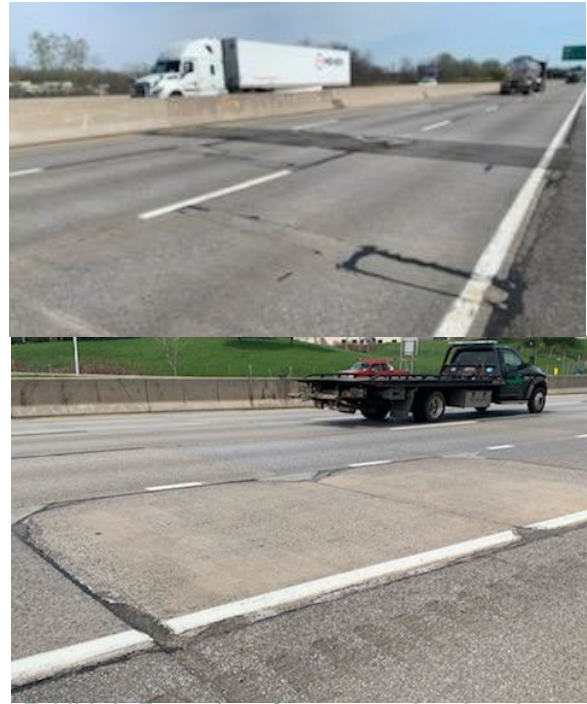
Exhibit 2: Examples of pavement deterioration on this segment, with extensive patching and repairs
